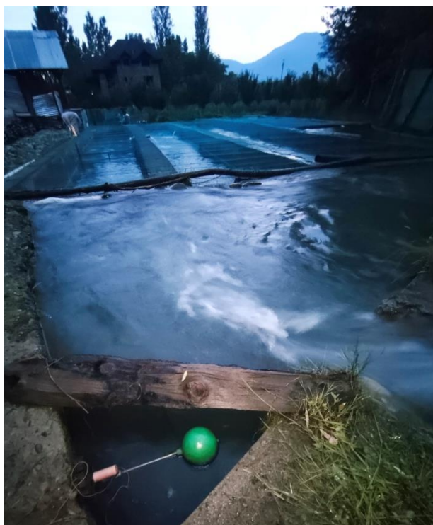
Water siren system installed at Royal Rainbow Trout Fish Unit, Sallar Bhagwani, to monitor and alert for consistent inlet water flow into the raceway, ensuring uninterrupted aquaculture operations.
